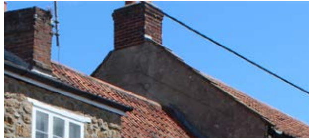
Clay tile roof with brick chimney, hipped away from the street but at varying heights within the terrace.
