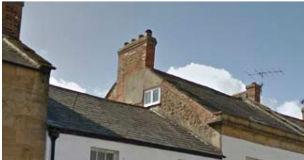
Slate roof with brick chimney. Coping stone, stone soffit and fascia features.
