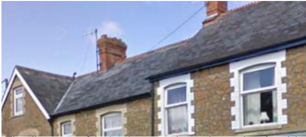
The linear roof is broken up through a mix of gable ends and is stepped due to the topography.
