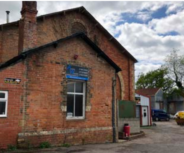
Dilapidated and unkempt frontages
