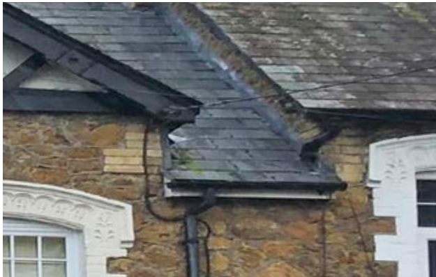
Slate roof and gable feature above the windows. Windows have traditional painted detail surrounds.
