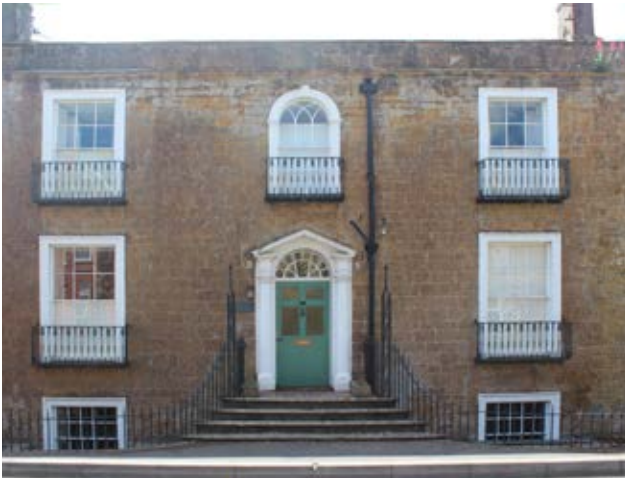
Large imposing Georgian villa with a marginal set back. Respectful relationship with topography.
