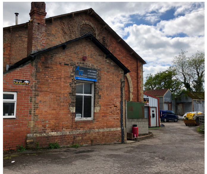
Dilapidated and unkempt frontages
