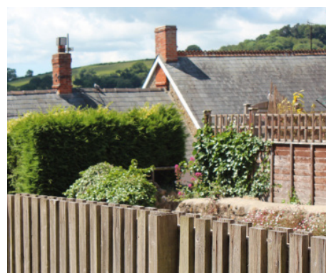
The topography allows close up and direct views of roof tops, features and chimneys.
