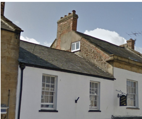
Slate roof with brick chimney with coping stone, stone soffit and fascia features.
