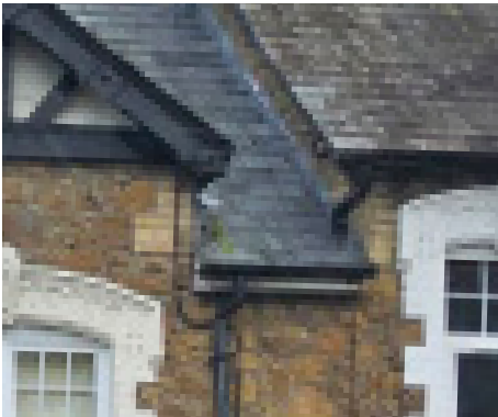
Slate roof and gable feature above the windows. Windows have traditional painted detail surrounds.
