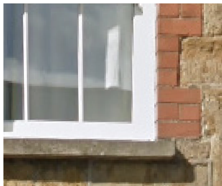
Traditional natural stone building with brick detailing, stone sill and sash windows.
