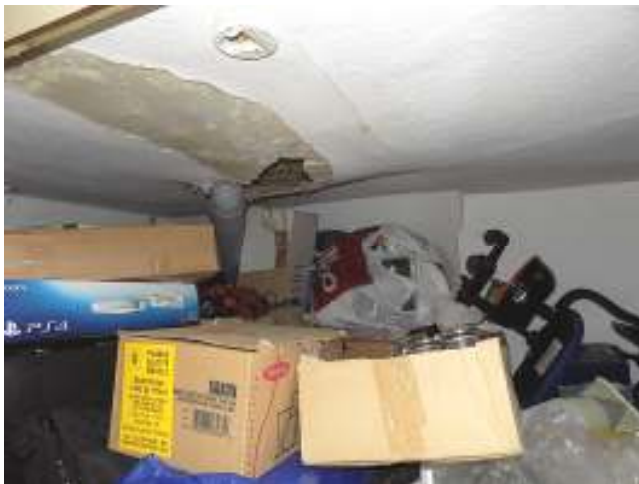
Collapsed ceiling above bathroom
