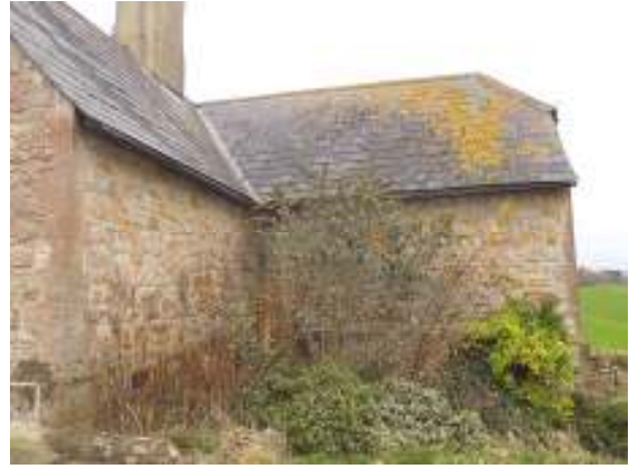
Moss to roof slope
